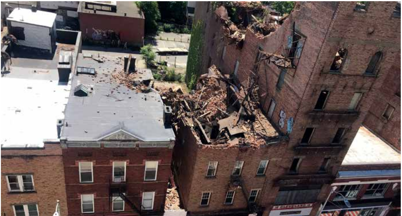
The top of 19 Academy St. in the City of Poughkeepsie collapsed dropping debris and causing damage at other properties. Ryan Santistevan/ Poughkeepsie Journal
