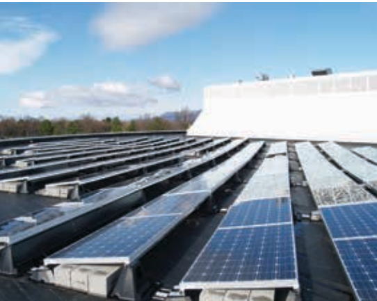
Solar panels atop the roof of Elting Gym
